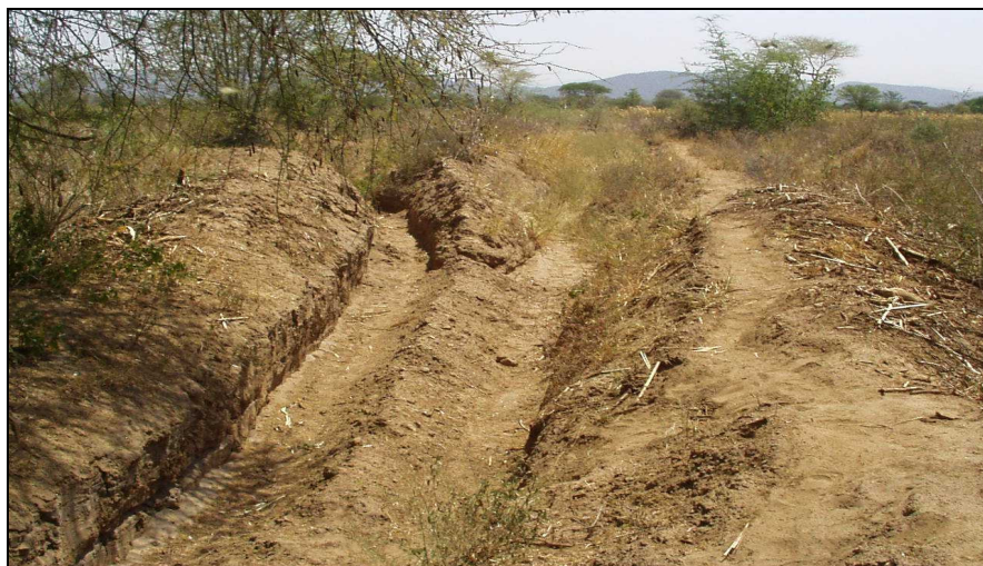
Ethiopia – typical flow division between two tertiary channels
